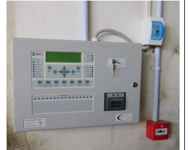
Fire Detection system
